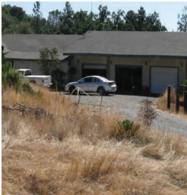
DEFENSIBLE SPACE NONCOMPLIANT
